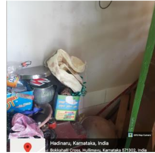
Toilet being used as storeroom in New Bokkahalli
