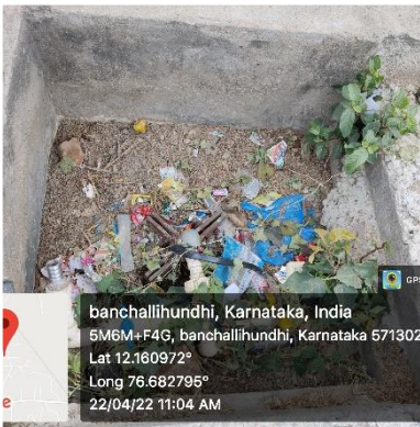
Borewell being used as dump site in Bachallihundi
